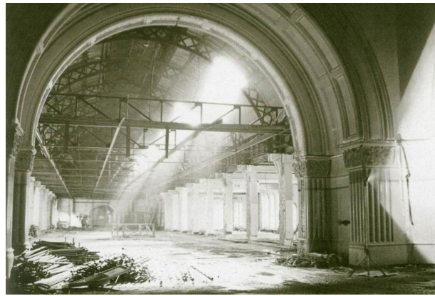
Figure 66 –The top floor at the commencement of works in 1984. The structure which supported the false ceiling under the barrel vault is evident and the concrete infills of the gallery voids had yet to be removed. Sheets of corrugated iron which replaced the original glass had been removed to allow light to be admitted
