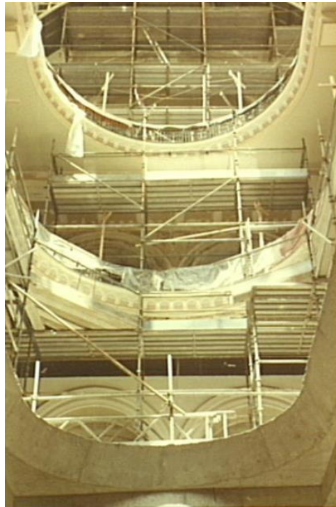
Figure 75 - Looking up through the newly recovered central dome area prior to the installation of Source: City of Sydney Archives, SRC11048
