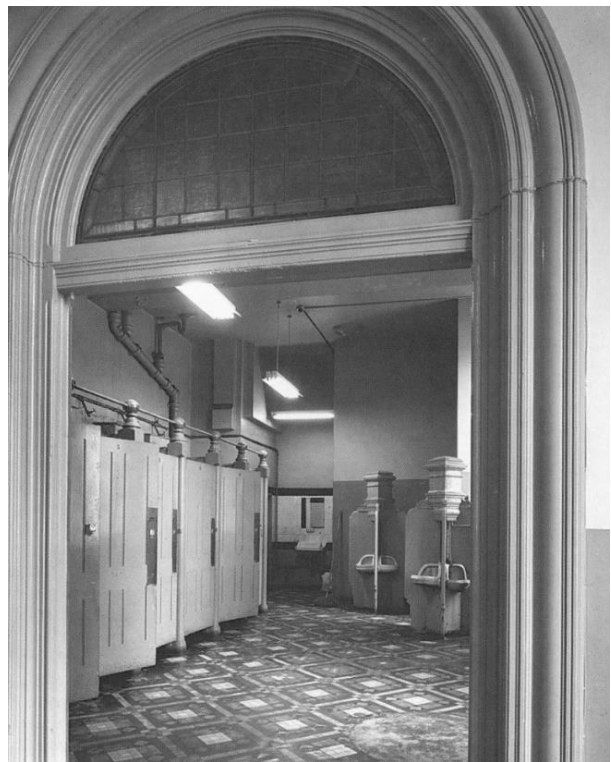
Figure 68 –Some of the men's bathrooms with their cast iron and porcelain urinals and partition posts were amongst the few internal areas to remain moderately intact
