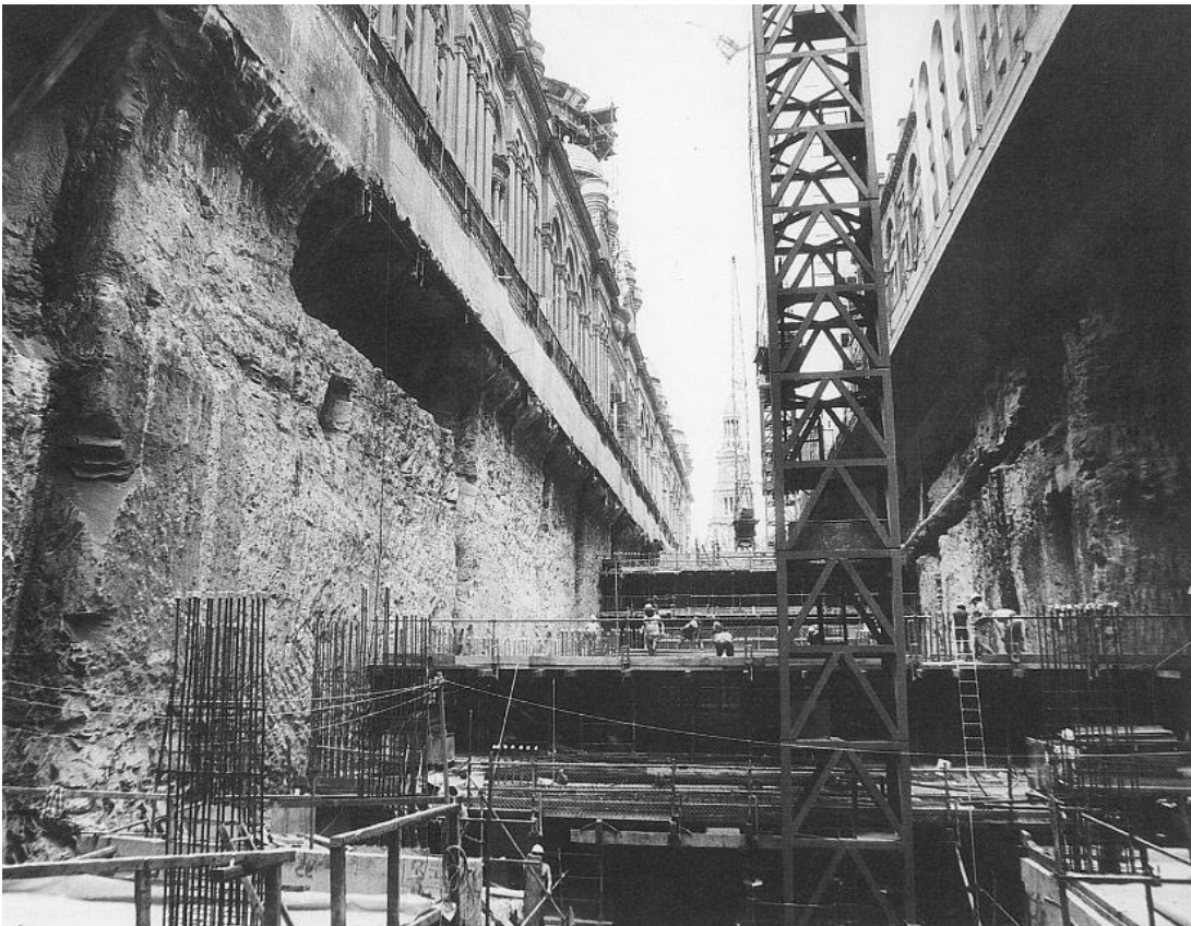
Figure 72 – Excavation for the car park, the QVB can be seen perched on the edge in the top left of frame
